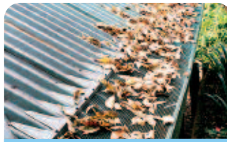
Mesh suspends leaves above gutters & wind blows them away
