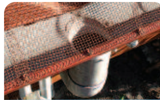
Sunlight and wind dries out gutters completely
